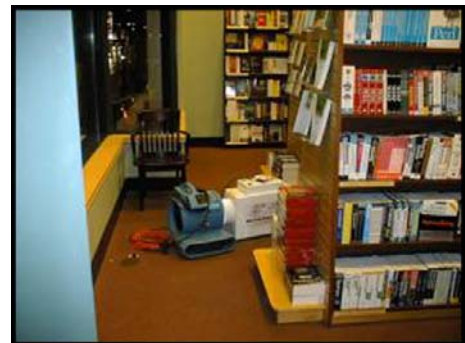
Figure 2 Elimination of Mold Due to a Water Leak at a Library
