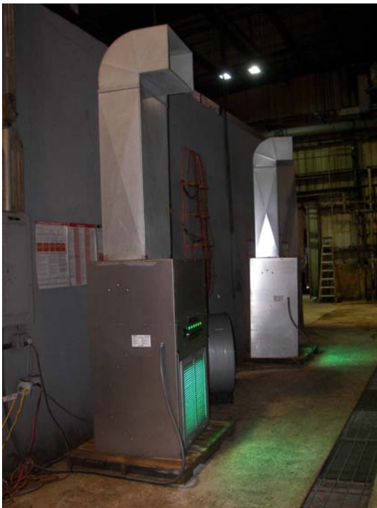
Figure 4 Rendering Plant Test Installation
