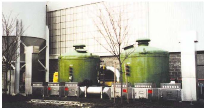
Figure 3 Wastewater Plant Odor Control
